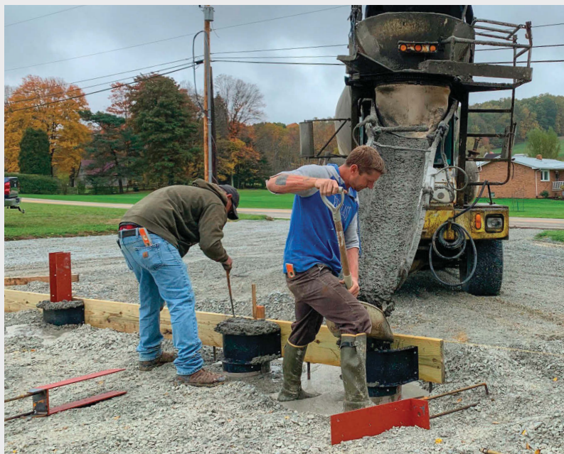
Pour footings. We used my skid steer equipped with an 18-in. auger to drill the building's 48-in. deep footings, adding up to 10 yd. of concrete. A pressure-treated 2x10 holds the above-grade plastic form and contains the concrete slab to be placed and finished later. Rodding the concrete footing with a piece of rebar prevents voids.
